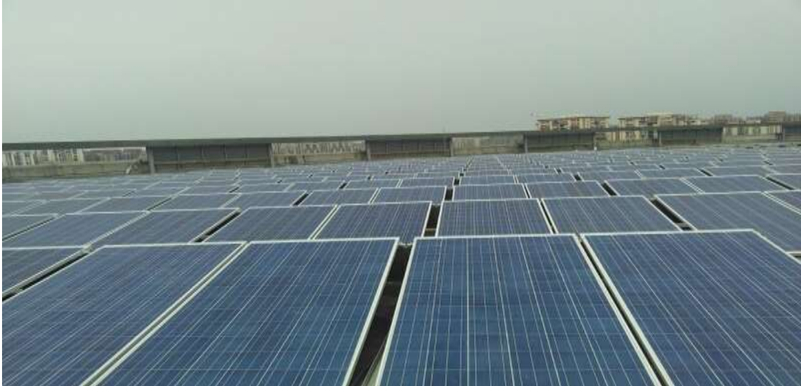
Solar PV Power panel
