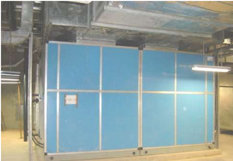
Air Handling Unit
