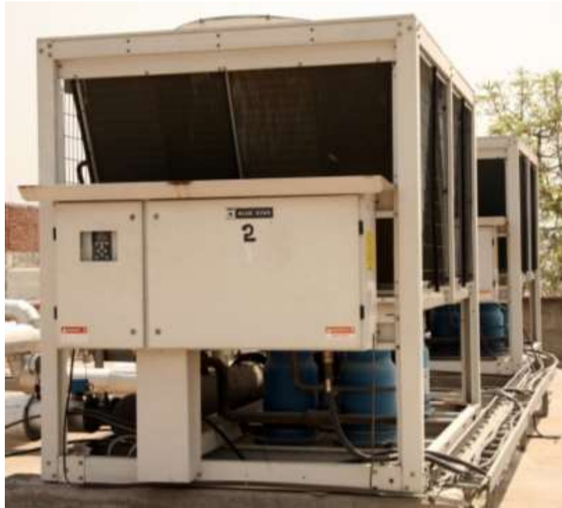
Air Cooled Chiller
