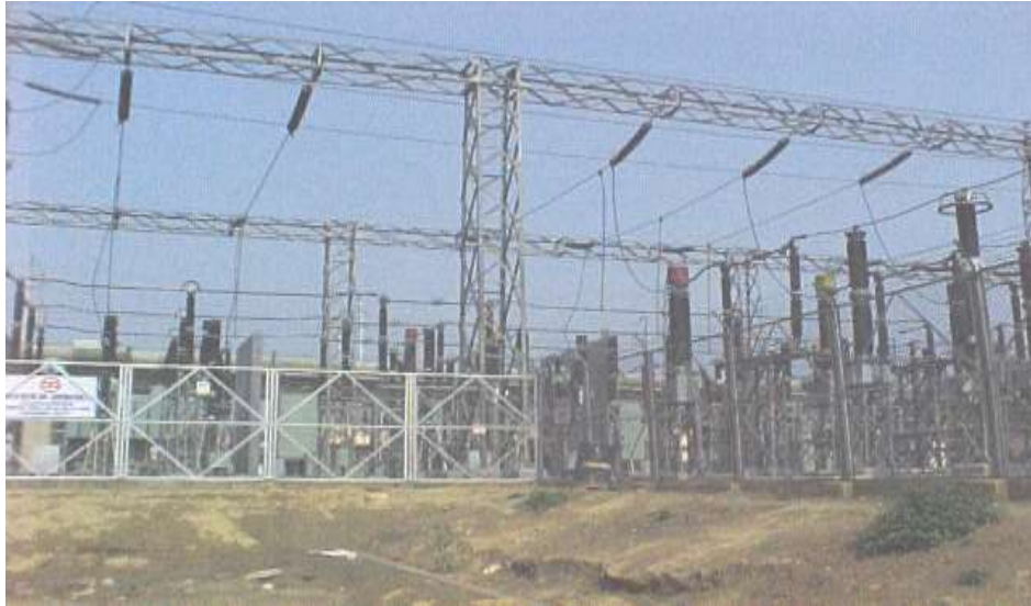
Typical High Voltage Receiving Sub-station
