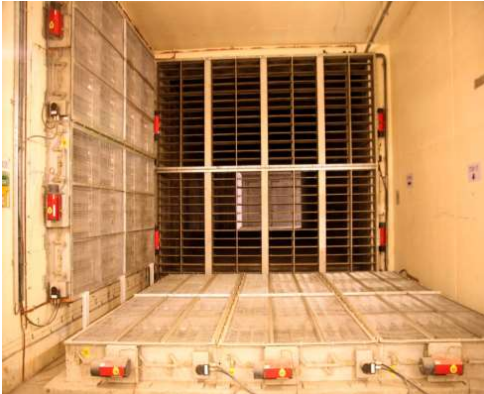
Tunnel Ventilation Dampers
