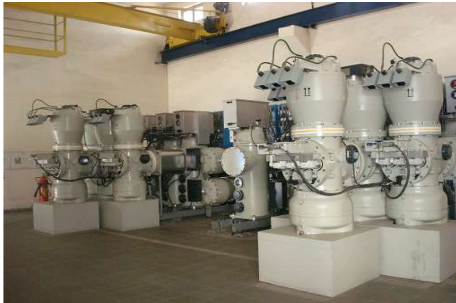
Typical High Voltage Gas Insulated Sub-Station (GIS)
